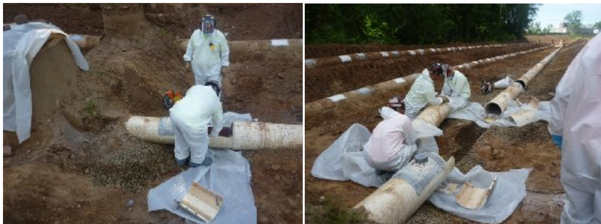
Photos 4 and 5. Characterization of buried piping.
