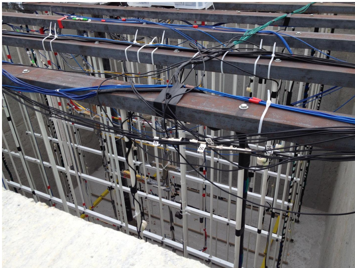
Figure 2. Sensor Installed on Panels. As designed, many sensor PIs had to install sensors on multiple panels in order to have a sensing grid throughout the cube volume.
