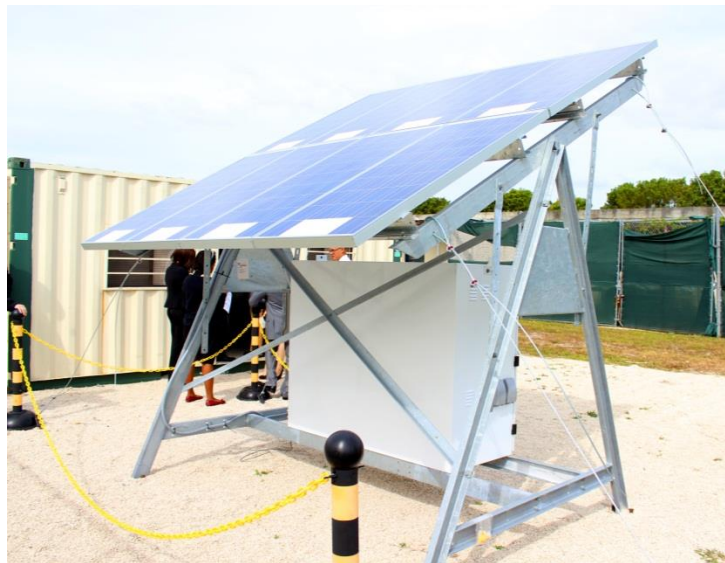
Figure 19. Photovoltaic System installed near the MSTB in order to power the sensor systems during energy analysis.
