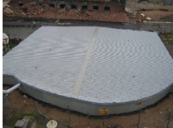
Figure 8 – Temporary weatherproof cover installed in 2004 had a stabilising effect on radiation levels
