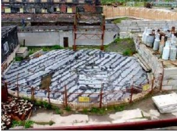
Figure 7 – Concrete beams and bitumen asphalt over DSU 3A covered provided poor weather protection
