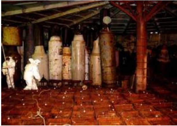
Figure 9 – Inside DSU 2A. Radiological conditions meant only brief access was allowed
