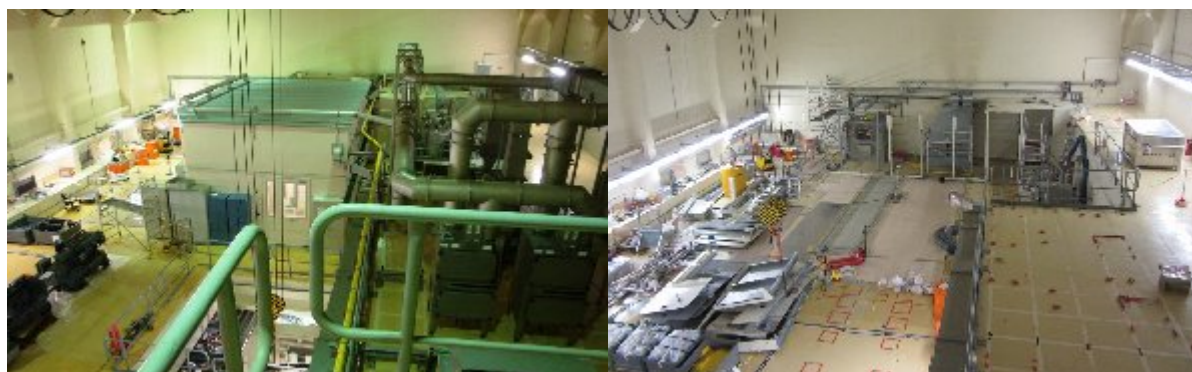
Fig. 5. HLLW storage building crane hall before and after dismantling of the HA laboratory
