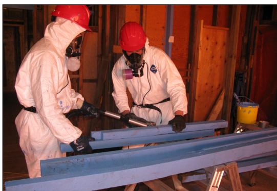
Fig. 5. Reducing the size of materials prior to packaging (note HEPA vacuuming at cut)
