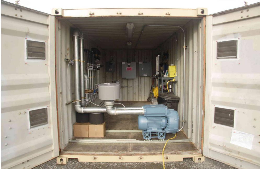
Fig. 3. Blower Package inside Container.
