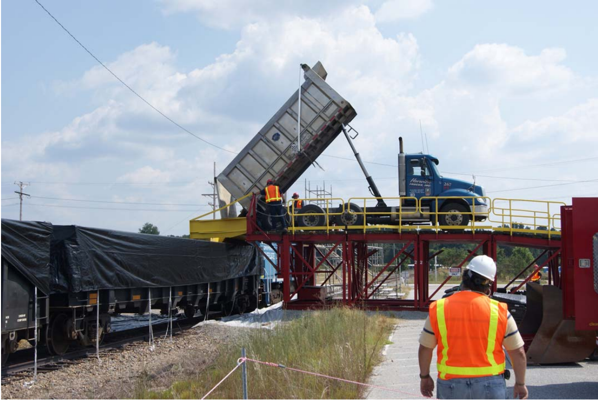
Figure 13. Loading of Rail Cars
