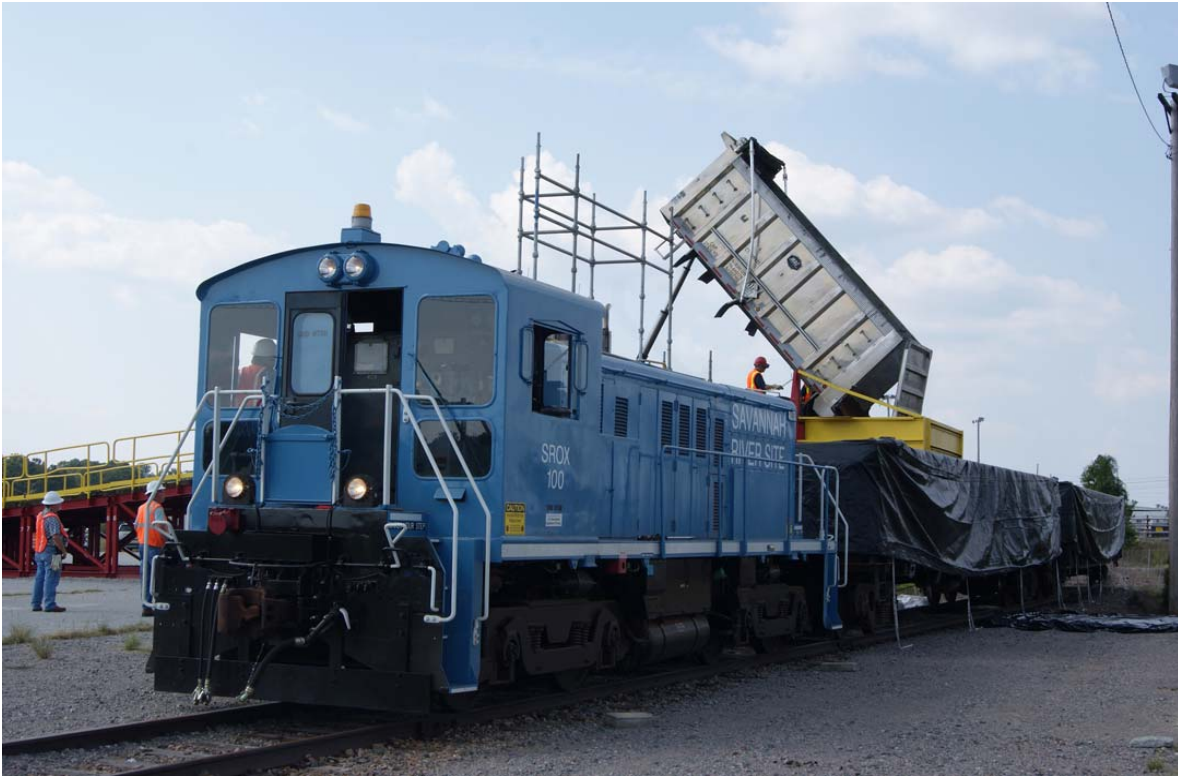
Figure 14. Loading of Rail Cars
