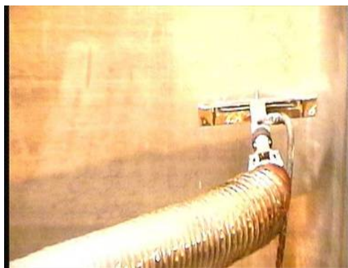
Fig. 5. Decontamination of the pit liner, using a spray ramp mounted on the robotic arm
