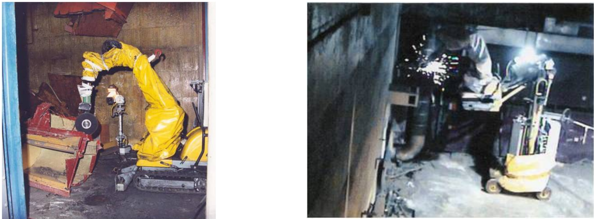
Fig. 8. Duct cutting in the filter room using EDA (left) and EDD (right)
