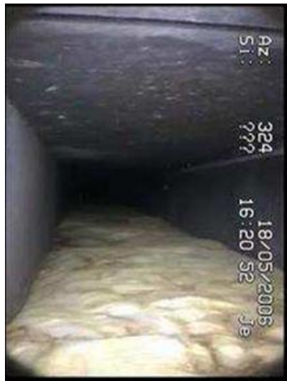
Fig. 1. Powder deposits inside the ventilation duct
