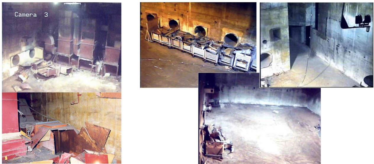
Fig.11. The space between filter room and the duct gallery before and after D&D operations
