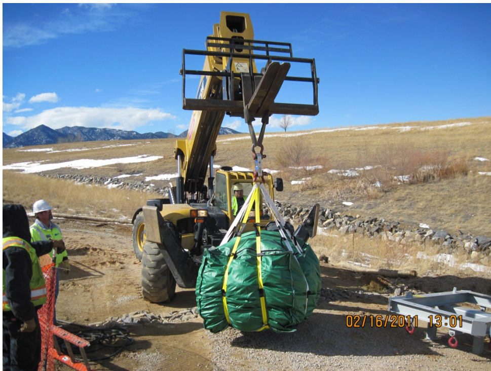
Figure 5. One of the 19 Super Sacks of spent MSPTS ZVI media being moved to a staging area for subsequent transport and disposal.
