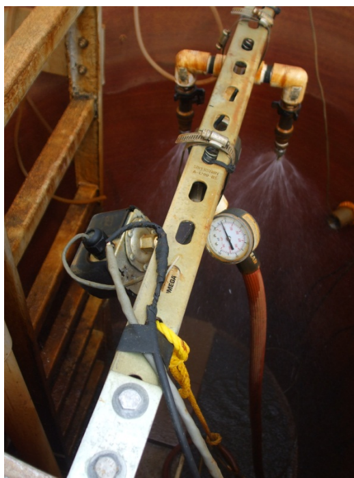
Figure 3. MSPTS air stripper spray nozzles in the effluent manhole.
