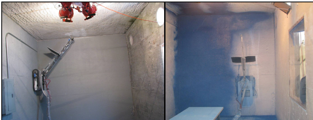
Fig. 4. ICM climber applying Promar 200 to ceiling (left) and PBS to wall (right).
