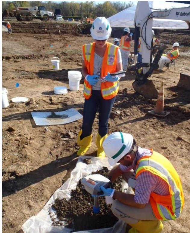
Figure 6: In-Field Use of InSpector 1000 for Nuclear Criticality Safety Measurements
