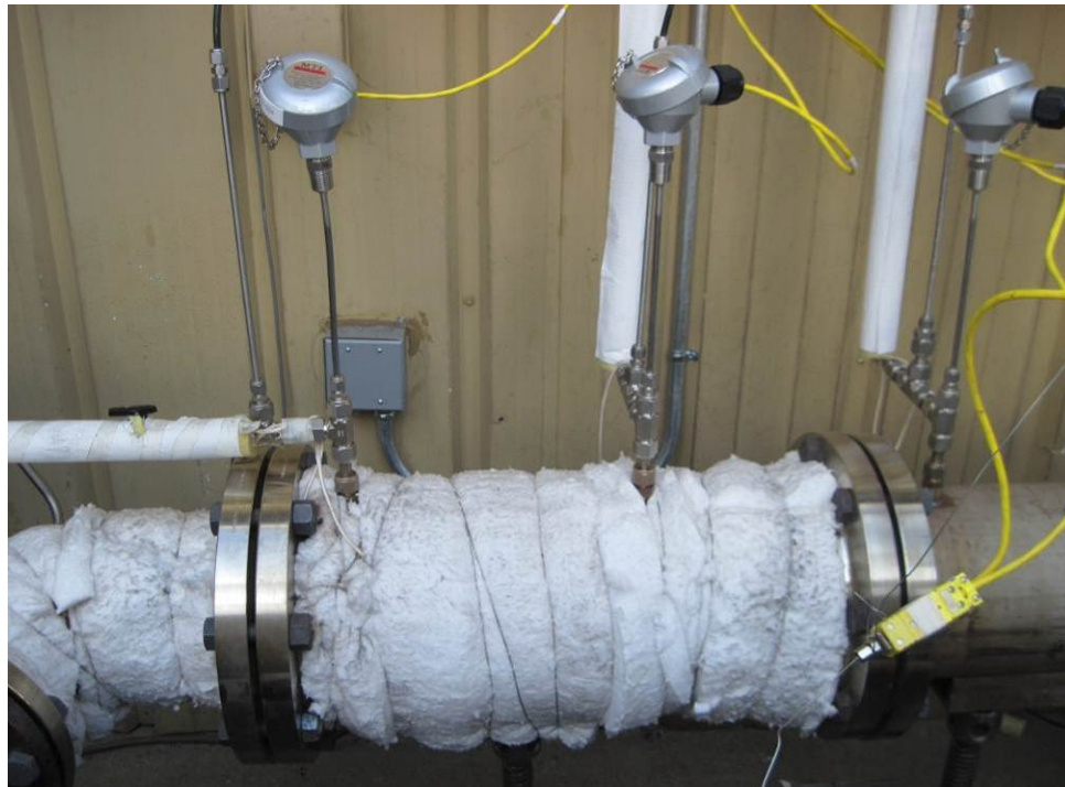
Figure 4. Photograph of the installed Catalytic De-NO x Unit.
