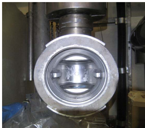
Fig.3 Interior surface condition (metallically clean) of a valve housing after ASDOC_D decontamination
