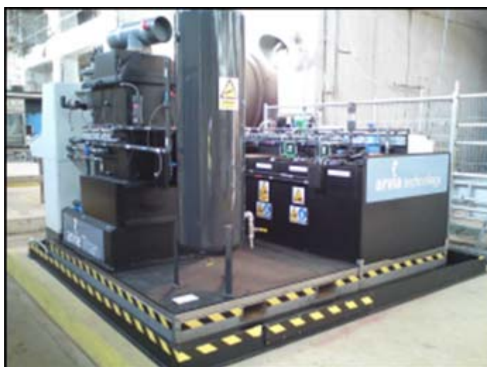
Fig 1. – Arvia Demonstration plant at Trawsfynydd
