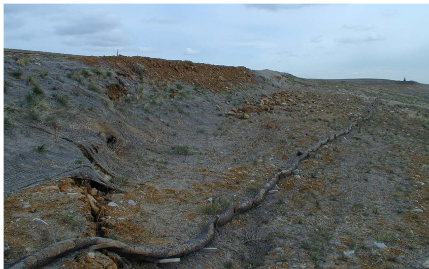
Figure 11. Cracking along downgradient side of the Original Landfill diversion berm.
