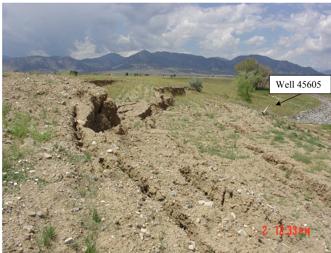
Figure 12. Hillside slump and cracking.
