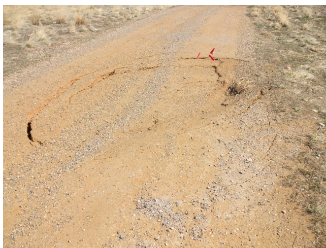
Figure 10. Depression and cracking in gravel road south of Building 771.
