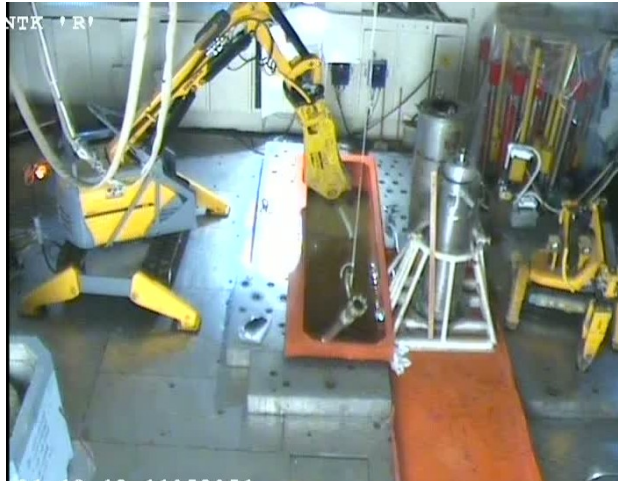
Fig. 5. A high-activity channel part being chopped off under water using remote-control Brokk mechanism.
