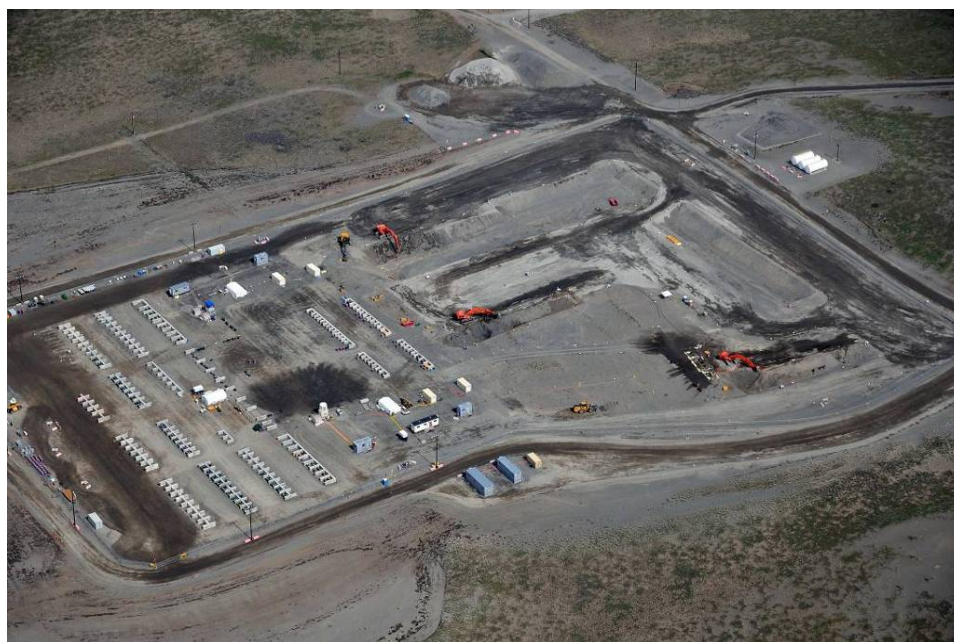
Figure 1. 618-10 Burial Ground Remediation, April 2012.
