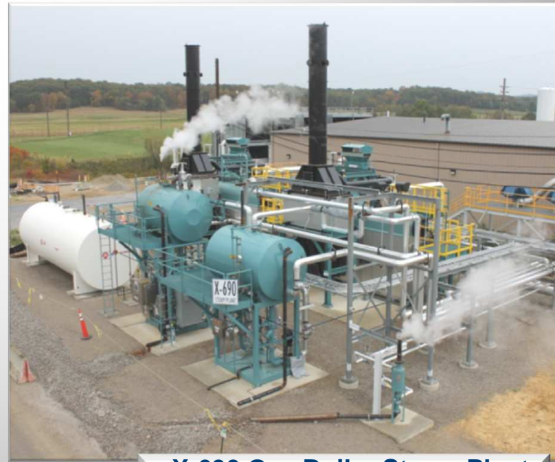
X-690 Gas Boiler Steam Plant
