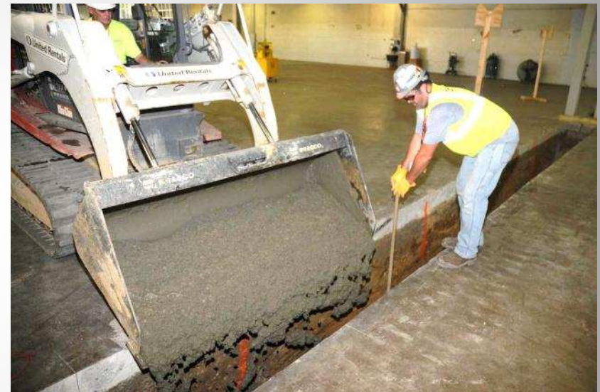
Measurements are taken to ensure the correct footer depth during the pouring of concrete for the new vault in the X-720 building.
