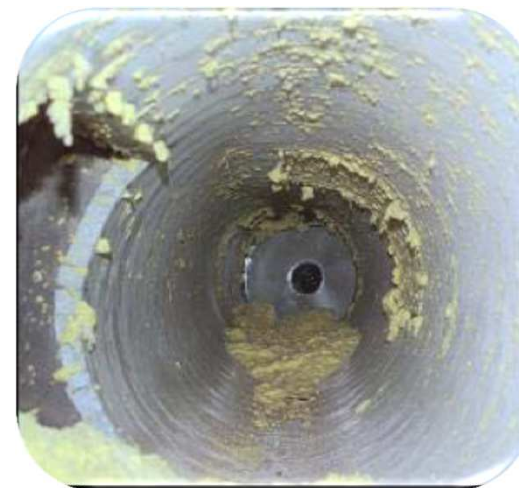
Contaminated duct awaiting D&D
