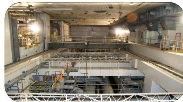
Heat Exchanger Pit @ - 6 m
