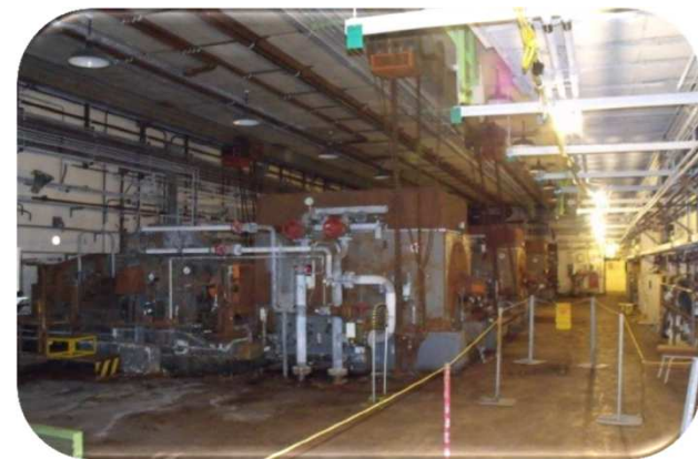
Pump Motor Room @ - 12 m
