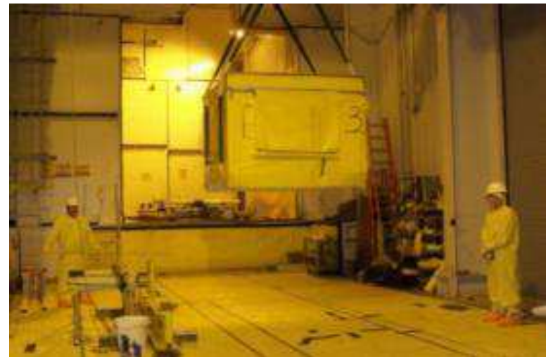
Removing B 25 Box of Low Level Waste in Remote-Handled Waste Facility (RHWF) Load Out
