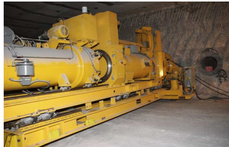
The Horizontal Emplacement and Retrieval Equipment (HERE) is used to push remote-handled transuranic waste into horizontal boreholes in the disposal room walls.
