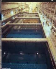
CPP-666 – Basin water storage
