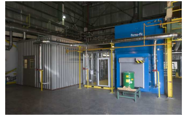
Tritium Treatment Enclosure
