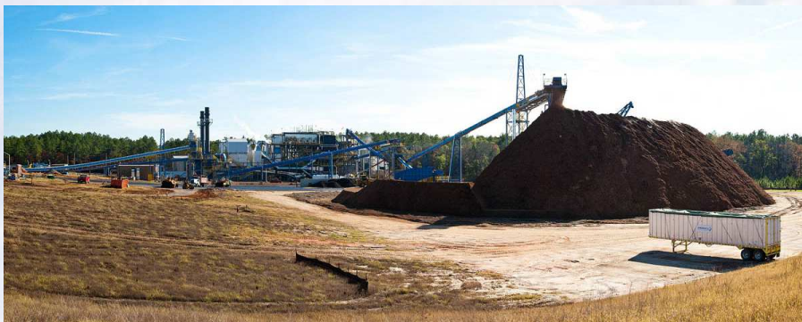
Biomass Cogeneration Facility at SRS, constructed and operated by Ameresco, began operations in December 2011
