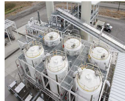
Hanford 200 W Groundwater Treatment Facility
