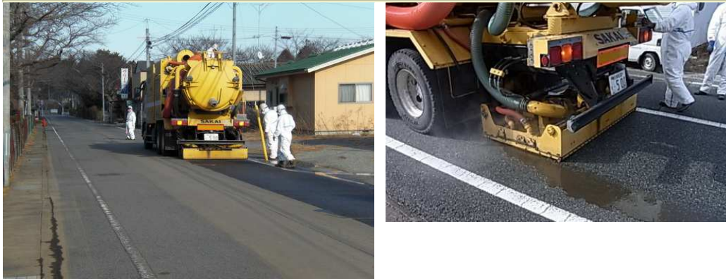
High-pressure water cleaning by vehicle for recovering functions of water drainage pavement
