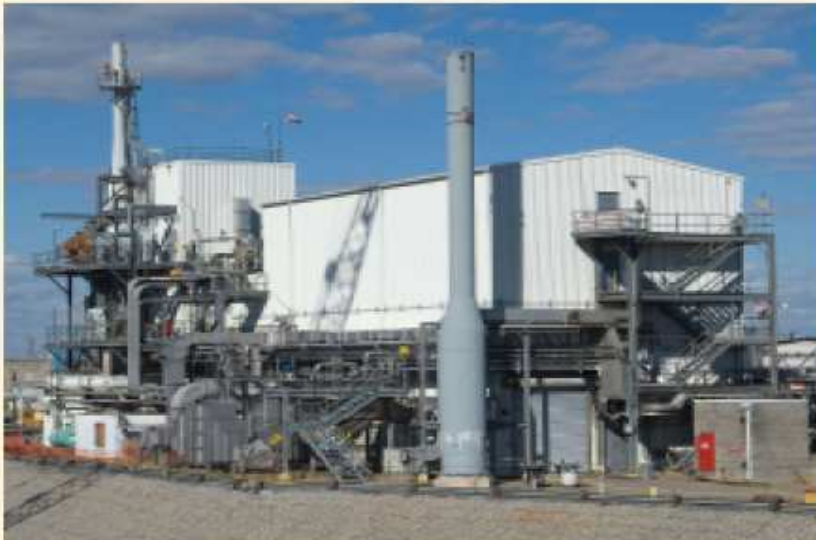
Actinide Removal Process (ARP)
