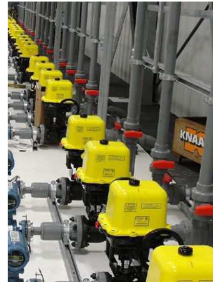
Equipment inside a groundwater treatment facility at Hanford.
