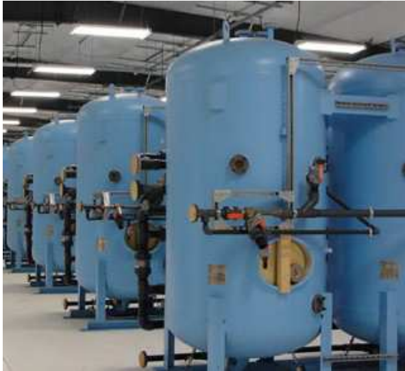
Tanks containing resins to remove contaminants from groundwater.
