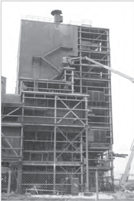
A crew removes cement-asbestos siding, left, from the 10-story portion of the Metals Plant.
