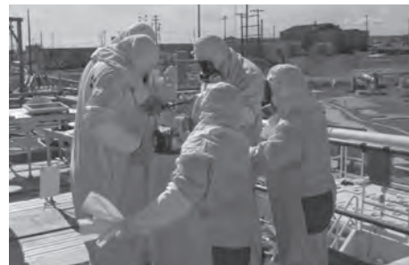
Standing near a pipe providing access to the tank below, workers initiate a water soak aimed at loosening hard-to-remove-waste from the bottom of C-109.
