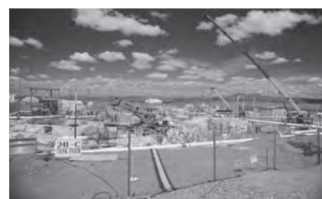
C Farm June 2012: ORP has successfully removed waste from a tenth storage tank at Hanford. Located in C Farm, C-109 is one of 16 underground tanks ranging in capacity from 55,000 to 530,000 gallons.
