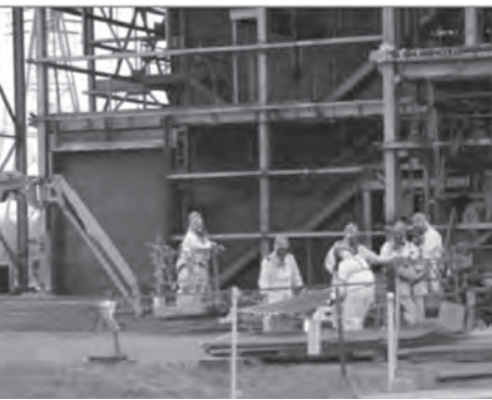
Workers package siding, above, so that it can be transported to the Paducah Site's industrial landfill.
