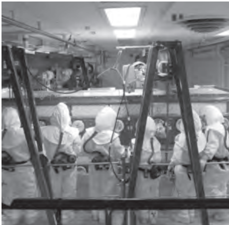
Workers in full protective and respiratory equipment install hoisting connections prior to initiating the lift to separate a 10-ton glovebox at the Plutonium Finishing Plant.
