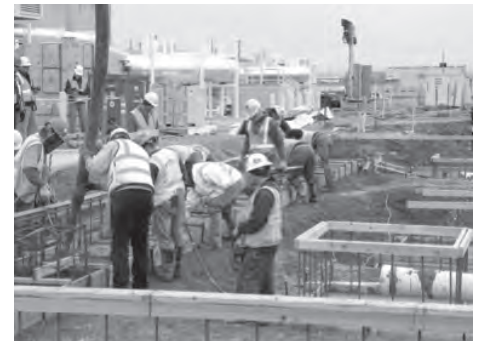
Workers are constructing an Annex that will support the sludge retrieval and transfer equipment at the K-West Reactor.
