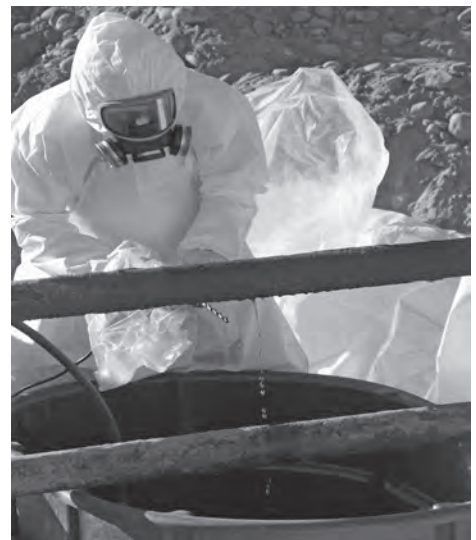
A worker cuts and drains pipe at a waste site in F Area. The pipe contained sodium dichromate, which was used as anti-corrosion agent.
