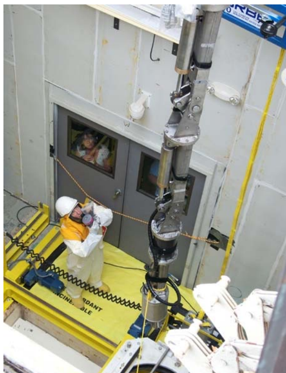
Figure 2: The robotic arm is lowered into the XCR through the roof hatch while an operator inside the XCR maintains radio contact with the mobile crane operations crew outside the MPPB.
