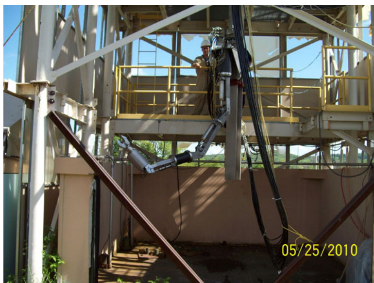
Figure 1: The NuVision robotic arm undergoes pre-deployment testing in the test tower at the WVDP.
