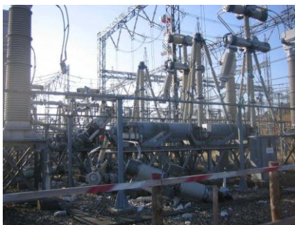
275kV Circuit Breaker of Substation
