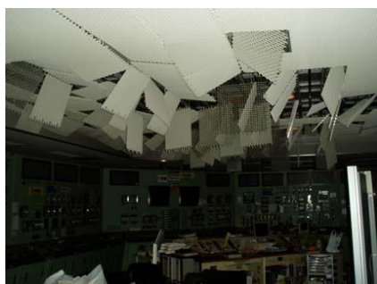
Main Control Room
