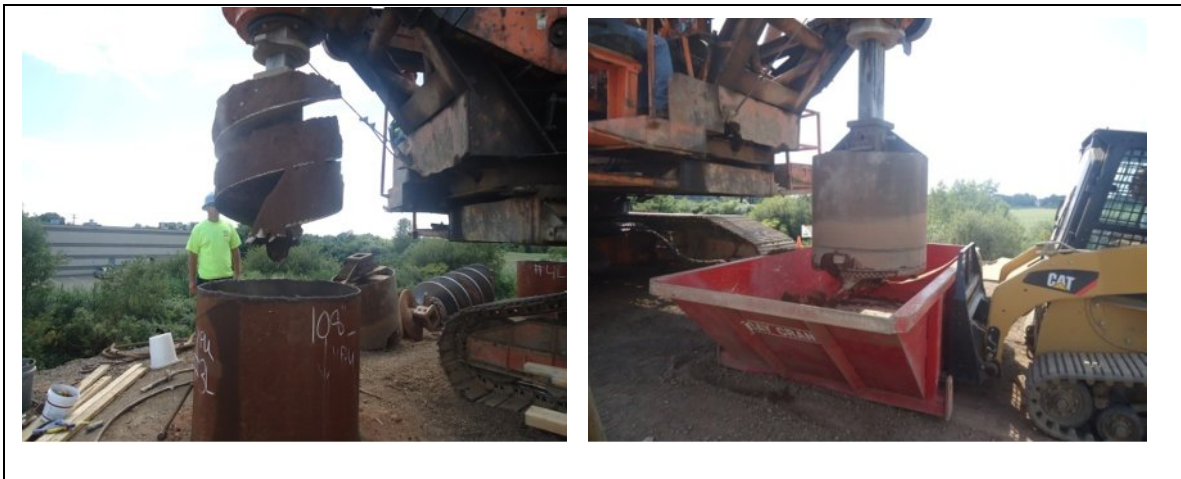
Figure 15. Removal by Rock Auger (Left photo) and by Bucket Auger (Right photo)
