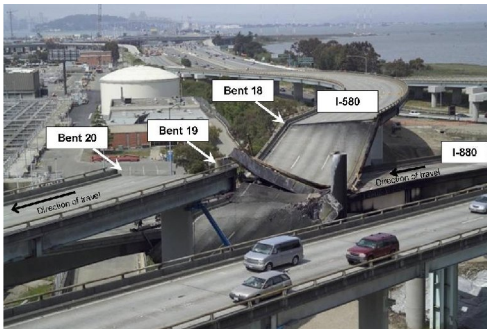
Fig. 2. Post-fire aerial view of the collapsed section of I-580 looking west. Picture from Caltrans http://www.dot.ca.gov/dist4/photography/images/070429 .
