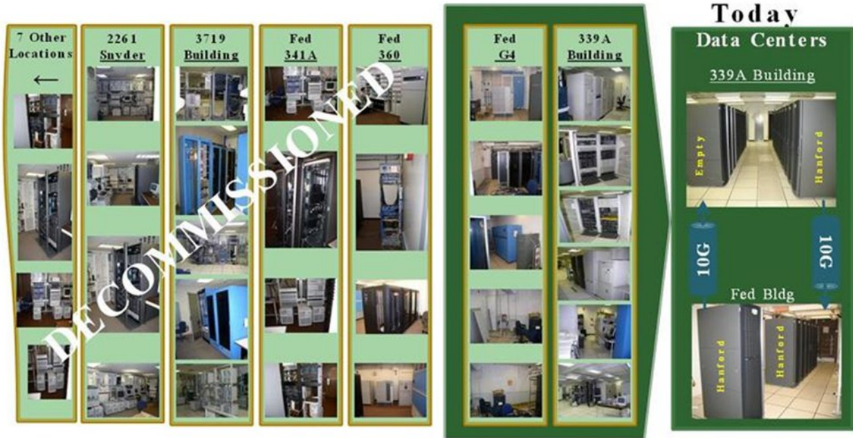
Fig. 2. Data center consolidation.
