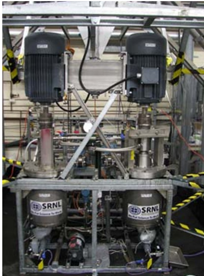
Figure 1. Dual Filter System Installed at SRNL
