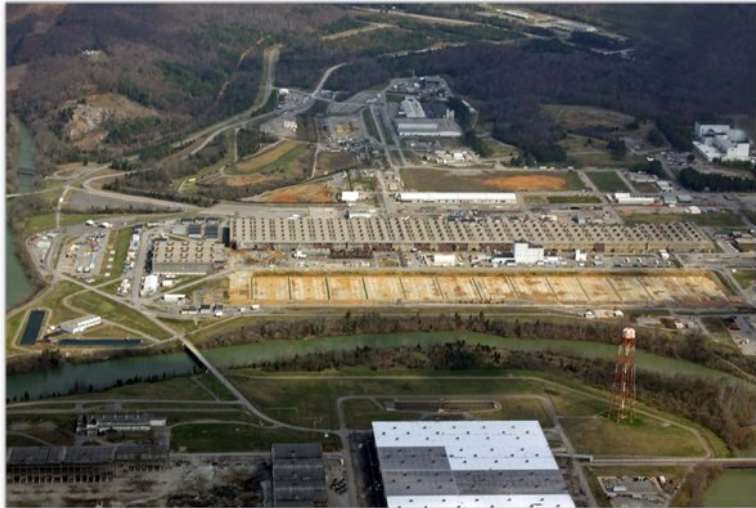
Fig. 4. West Wing Completion. Using the revised approach and control measures, the Bechtel Jacobs project team completed K-25 west wing demolition successfully, efficiently, and safely.
