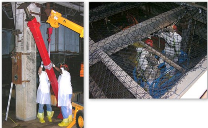
Fig. 2. Worker Protection. The project implemented new D&D approaches and structural reinforcement measures to mitigate the hazards resulting from building deterioration.
