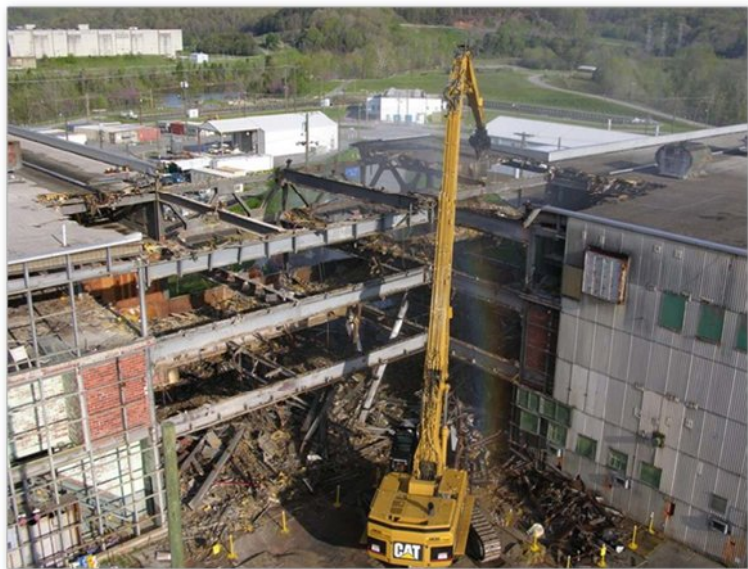
Fig. 3. Revised Demolition Approach. Once the project had demonstrated “criticality incredible” status, large equipment could be used to quickly dismantle the building without the need for additional controls.
