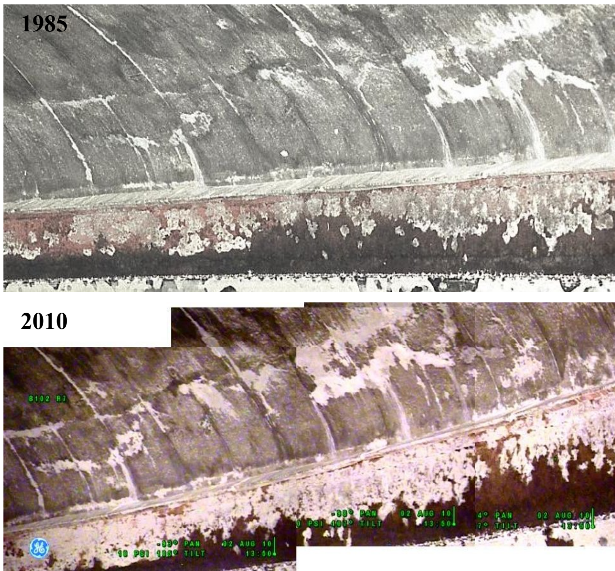
Figure 5. Comparative Photographs of Tank 241-B-102 Haunch Region
