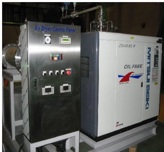
(a) Compressor and condenser
