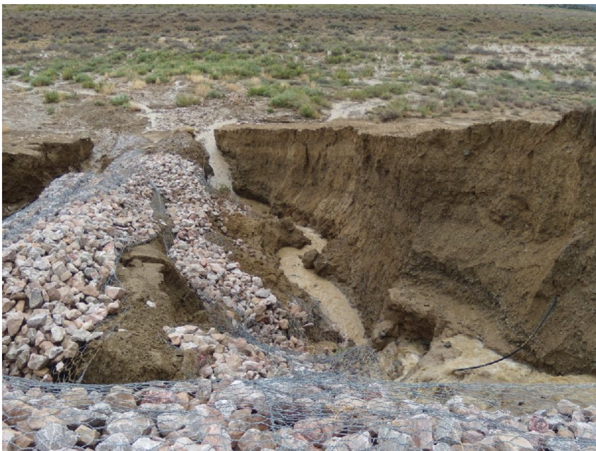
Figure 2. Storm damage to erosion control structure at L-Bar site.
