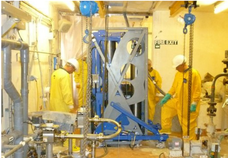
Figure 4: RDA in position in a resin vault plant room
