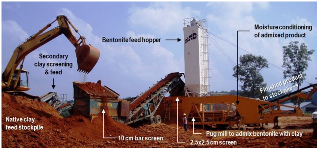
Fig 2. EMWMF used a pugmill for admixing bentonite with clay to produce superior quality material for the compacted clay liner.
