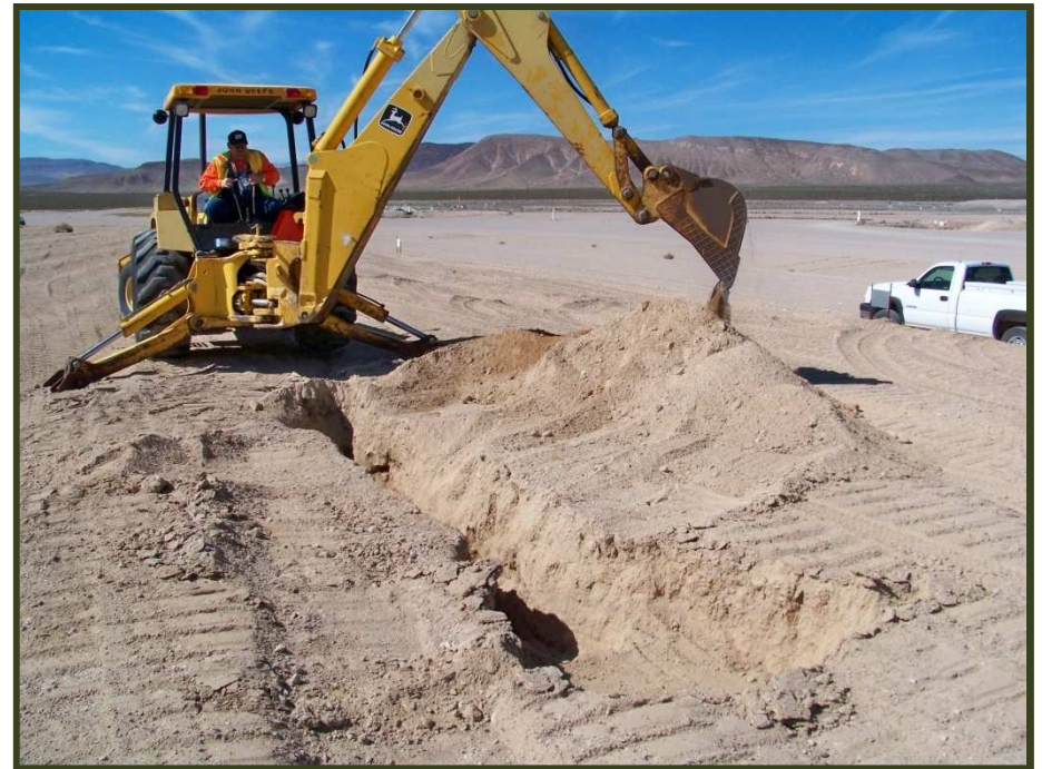
Completed MLLW Disposal Cell (18) at the Area 5 92-Acre Closure Monitored Independent Station Radioactive Waste Management Site (RWMS)
