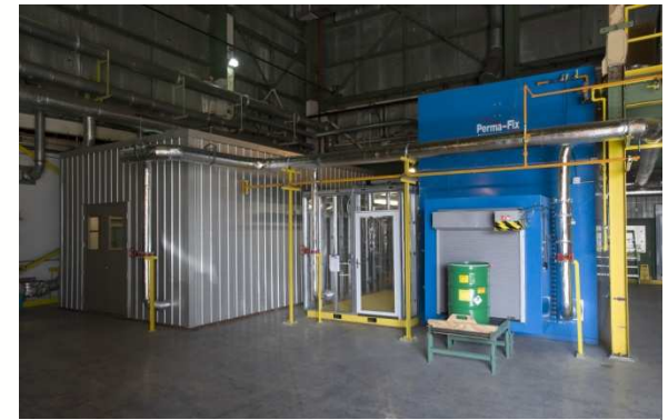
Tritium Treatment Enclosure
