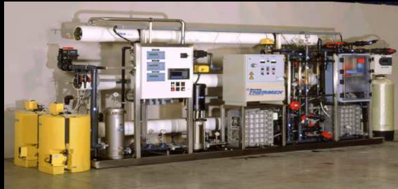
Liquid Waste Processing Equipment
