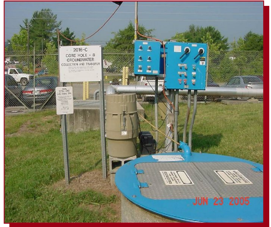
Groundwater collection system
