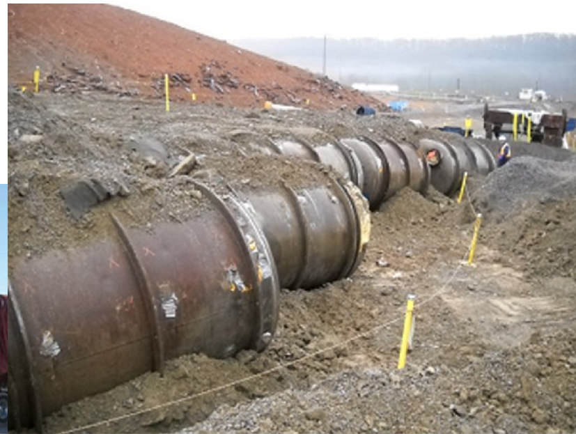
K-25 Converters shipped directly to EMWMF
