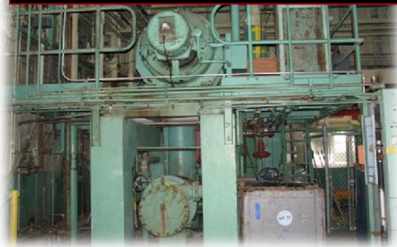
Homogeneous Reactor High Bay
