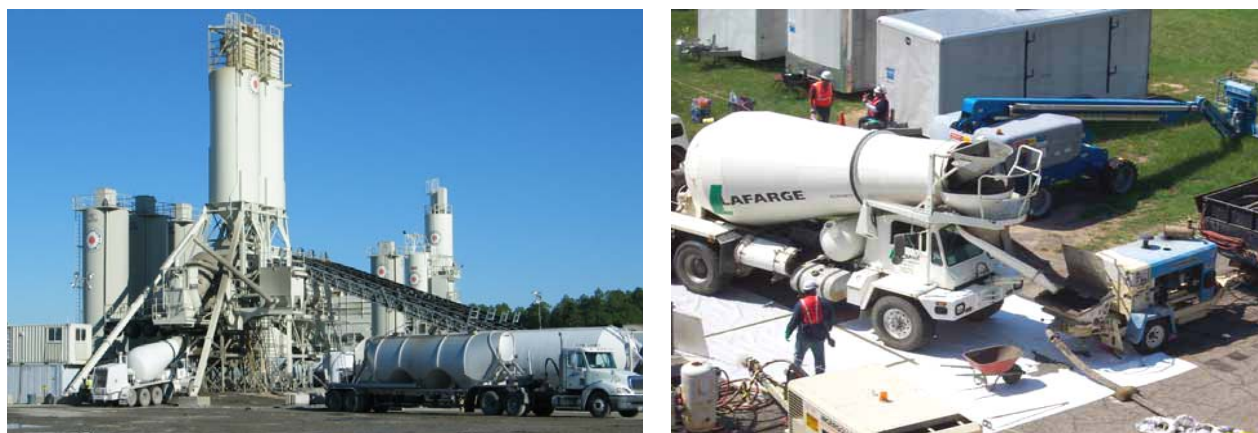
Figure 4. Two On-site Concrete Batch Plants Located in P-Area. Plants were used to produce ISD fill (left) and delivery and pumping of ISD grout in the R-Reactor Disassembly Basin (right).
