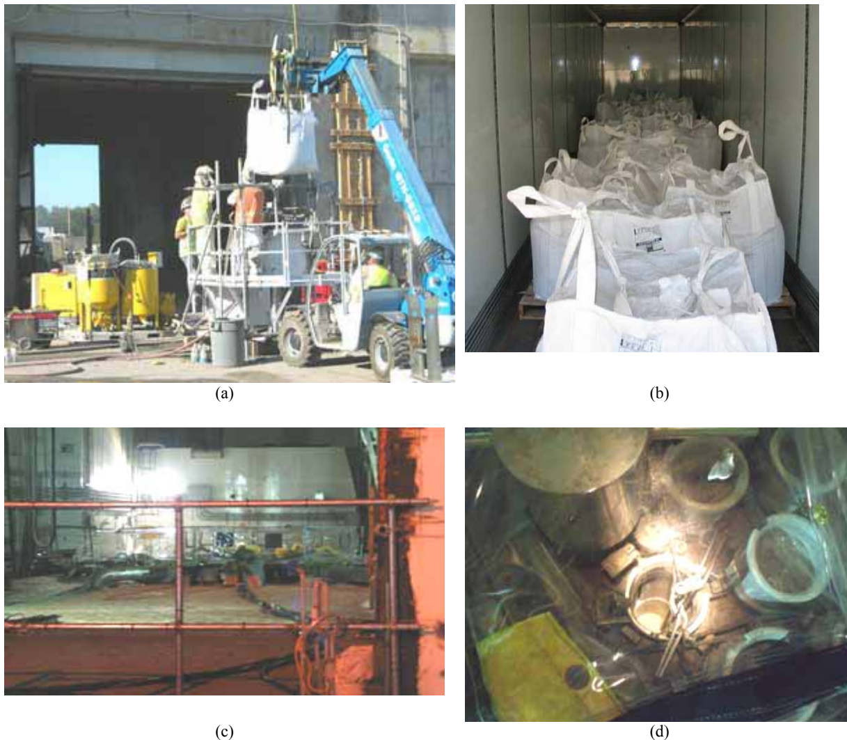
Figure 10. P-Reactor Vessel ISD. (a) grout production, (b) 2000 pounds of pre-blended grout delivered to P-Area in super sack, (c) view of reactor plenum with plastic containment hut and grout lines, and (d) view of filled P-Reactor Vessel – looking into opening with grout level about 16 inches from top working surface.
