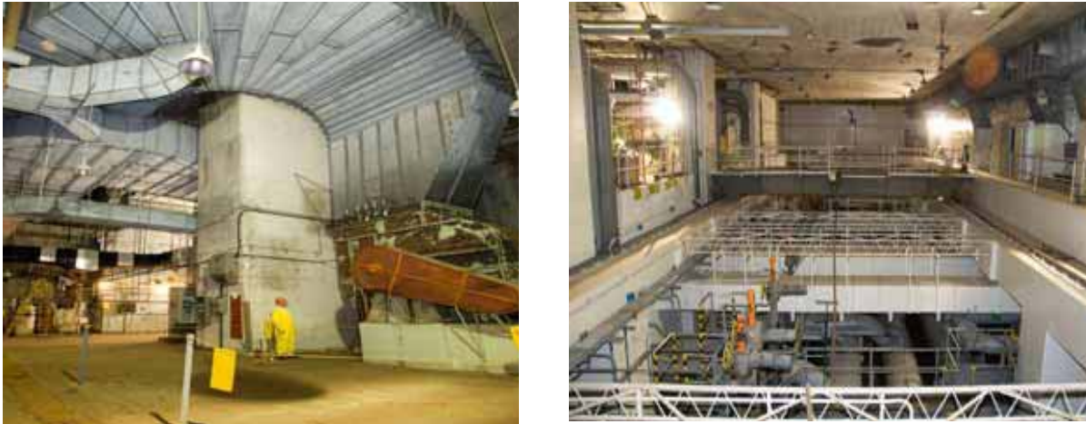
Figure 5. Examples of Rooms at the -20 and -40 Levels before ISD. Fan room at -40 level (left) and Heat Exchanger Pit at -20 level (right).
